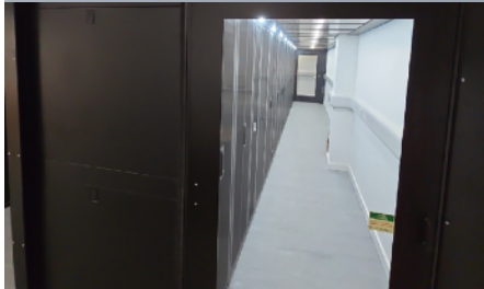
Enclosed hot aisle with in-row coolers
